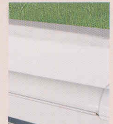
One-year-old Winnebago Industries fiberglass roof
