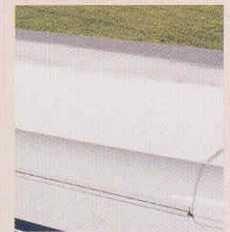
One-year-old Winnebago Industries fiberglass roof
