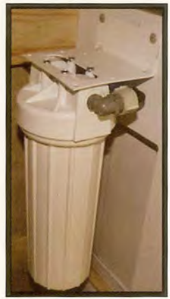
Water Filtration System
